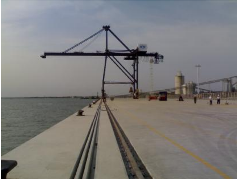
The first of 7 STS cranes of SITV in place at the newly installed Crane Rail System from MHE-Demag Vietnam and Gantrail.
