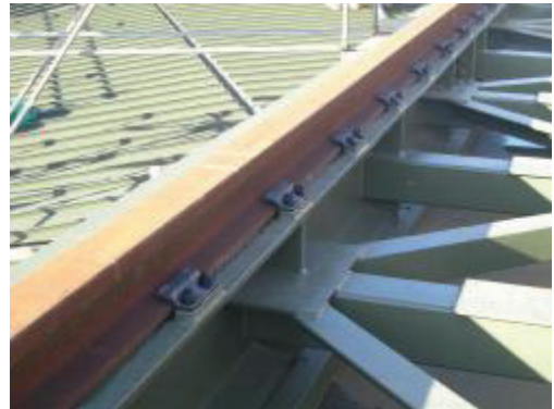
With one rail 'All clips are finally tighten after the rails are welded.'
